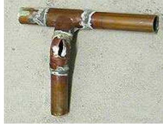
Damages by frost at water pipes
